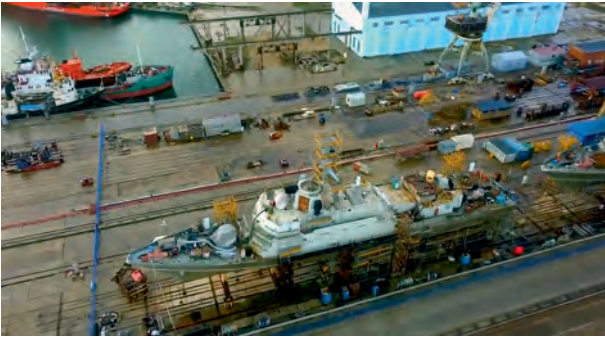
The Tsiklon missile corvette (yard number 801, Project 22800 Karakurt) is under construction on the open slipway at the Zaliv shipyard, a gun has been mounted, navigation equipment is being installed; the construction is proceeding as scheduled – it is expected to be completed at the end of 2020. The photo from the BlackSeaNews archive, February 2020
